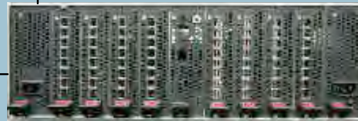
POE Router Rack
